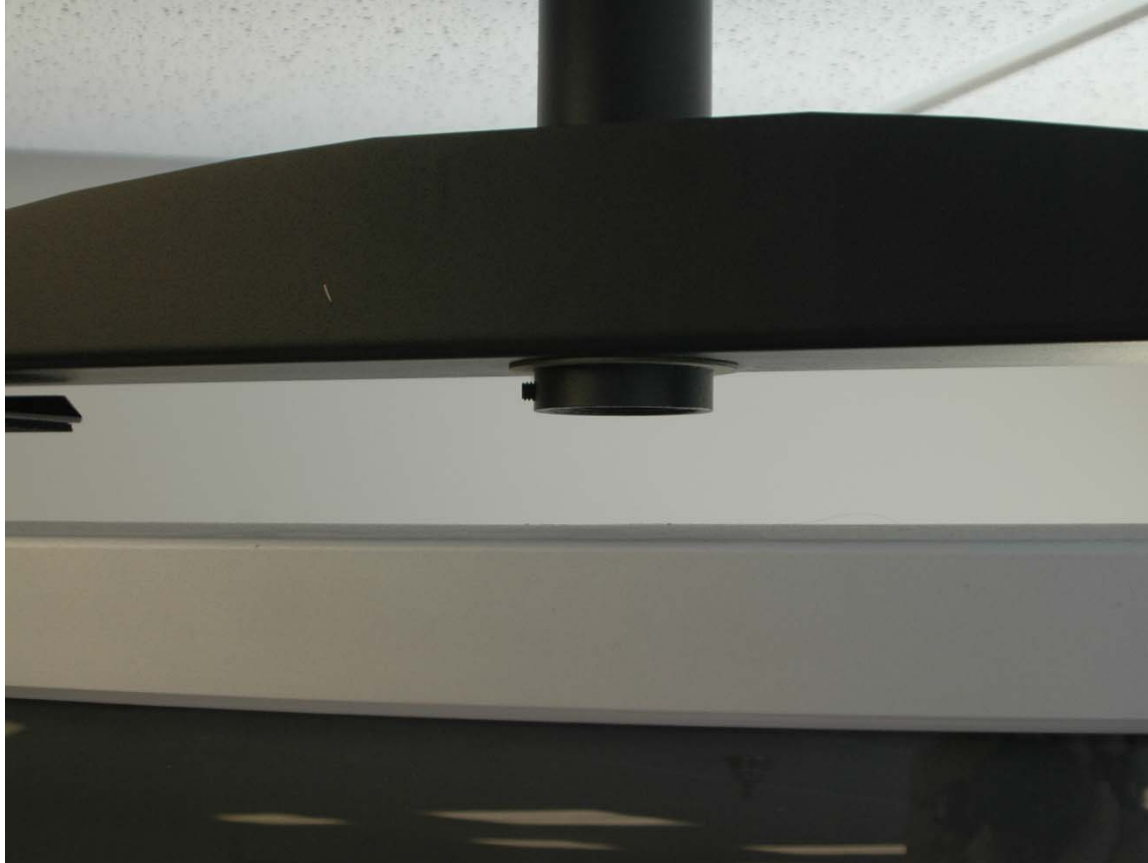
Bottom flange – incorrect installation
